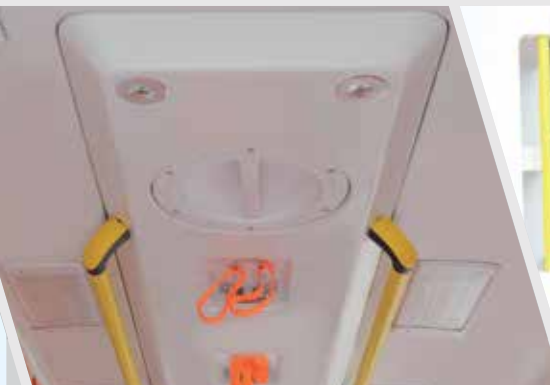
Glass fiber reinforced suspended ceiling, IV injection hook, exhaust fans
